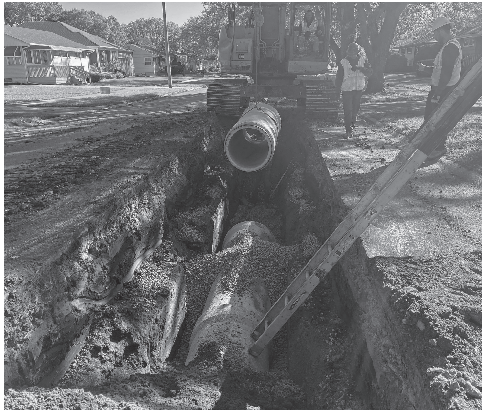
[ THE END OF LAKE LAVERNE ] Workers replace the old 12-inch storm sewers along Laverne Drive with lines that are double the size to reduce flooding. [photo provided]
